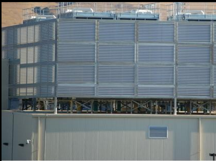
Old "Always ON" Chiller Design
